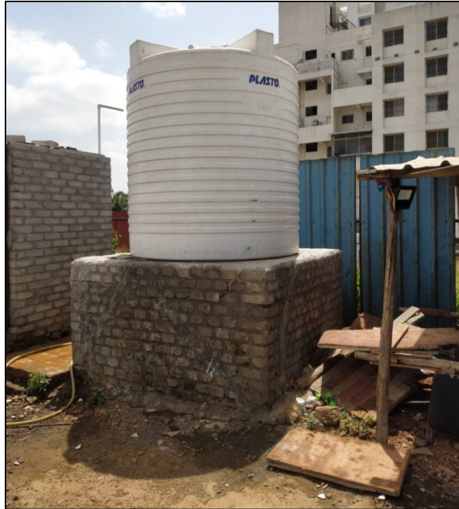
Drinking water facility for workers at site
